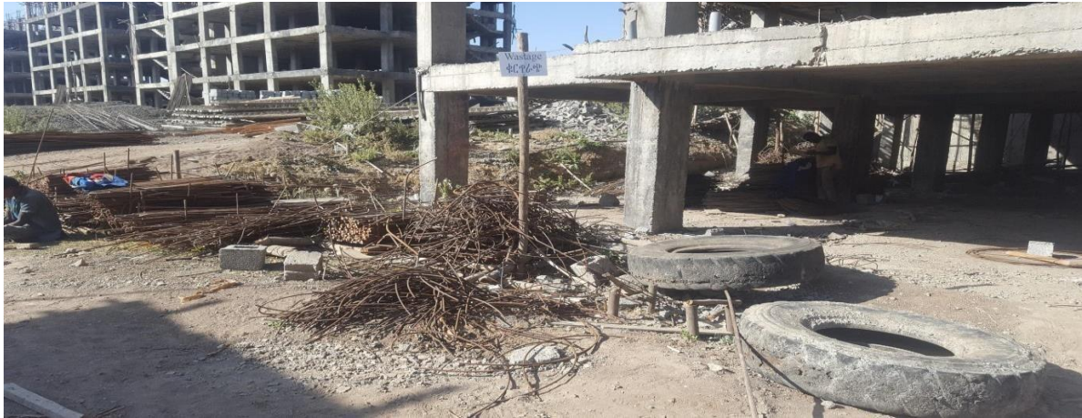
Figure 4.1 a, wasted reinforcement bar due to cutting problem
