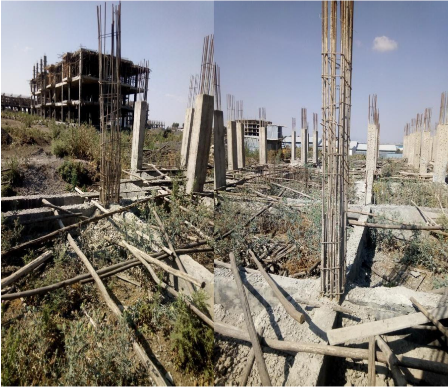
Figure 4.4 Demolished RCC columns due to poor workman ship
