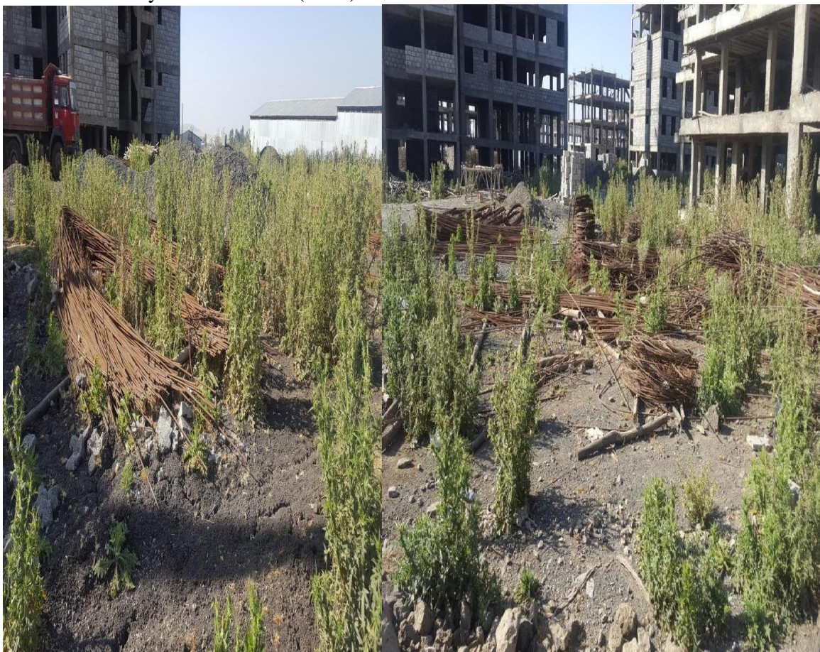
Figure 4.1b reinforcement placed in the wrong way
